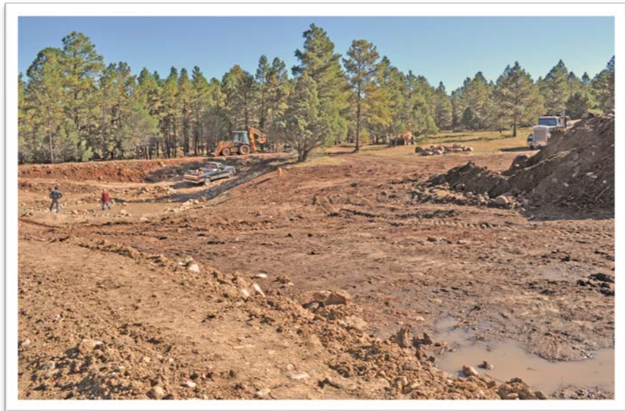
The pond cavity half excavated. Note the pile of rocks and large pile of reserved topsoil to the right of photo. (2010 Photo by J. Riddick)
